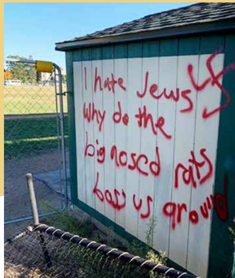
Antisemitic graffiti at George Washington High School in Denver, CO, photographed on October 18, 2021. Photo credit: James Stern
